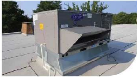
ROOF TOP PACKAGE UNIT
